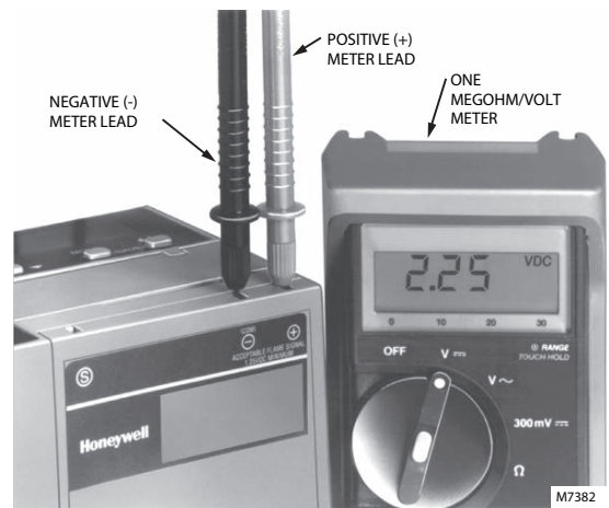
Fig. 11. Measuring voltage flame signal with 7800 Series controls.
