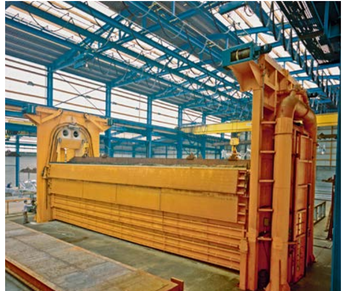
DH hoist units operating under arduous conditions in a galvanising plant
