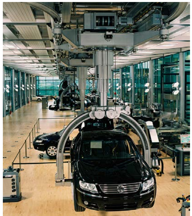
DH hoist units in the production line of a car manufacturing plant
