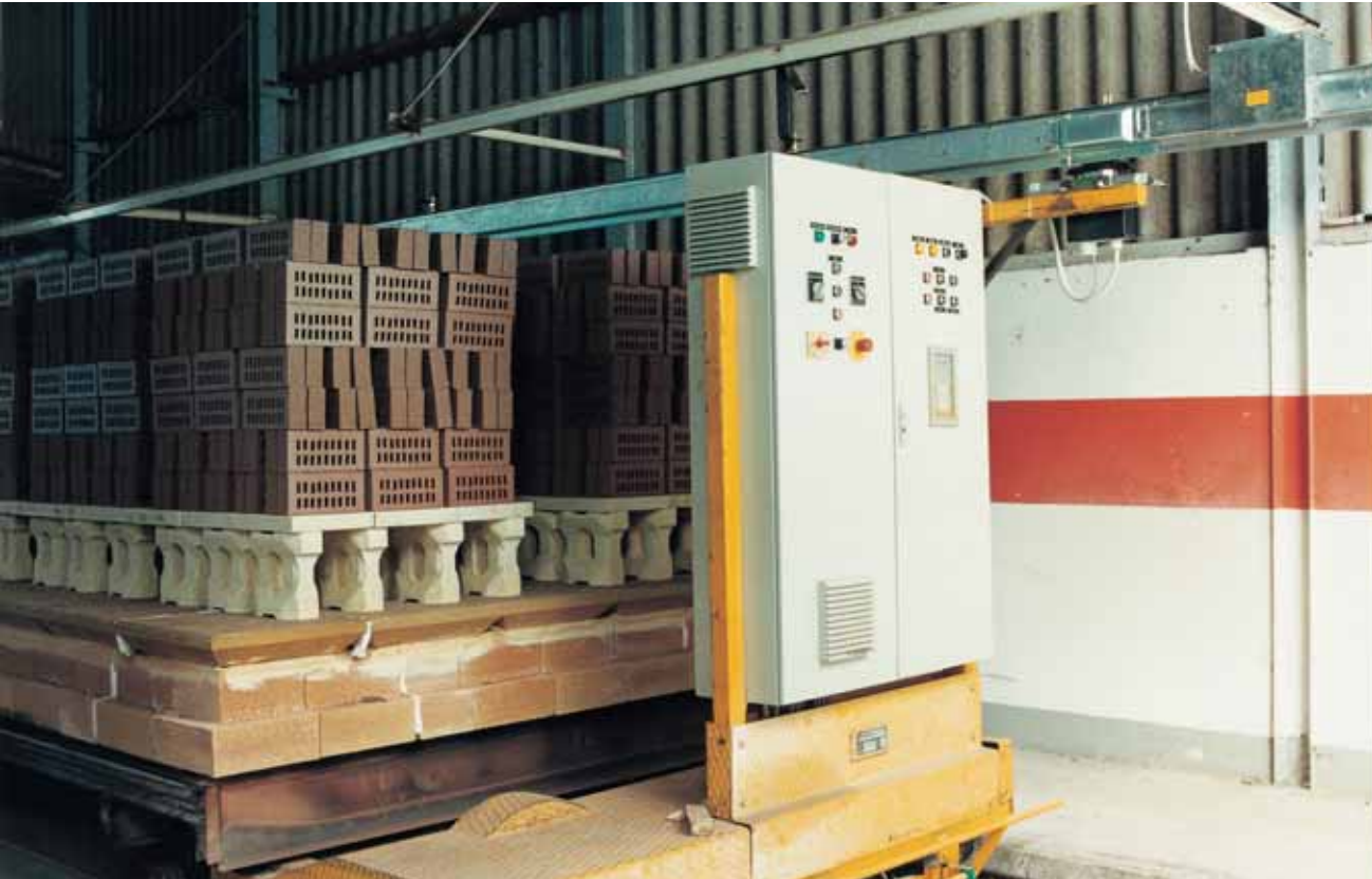
VAHLE POWERCOM®-data transmission at a brick kiln.
